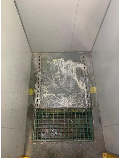
危废仓库集液池
